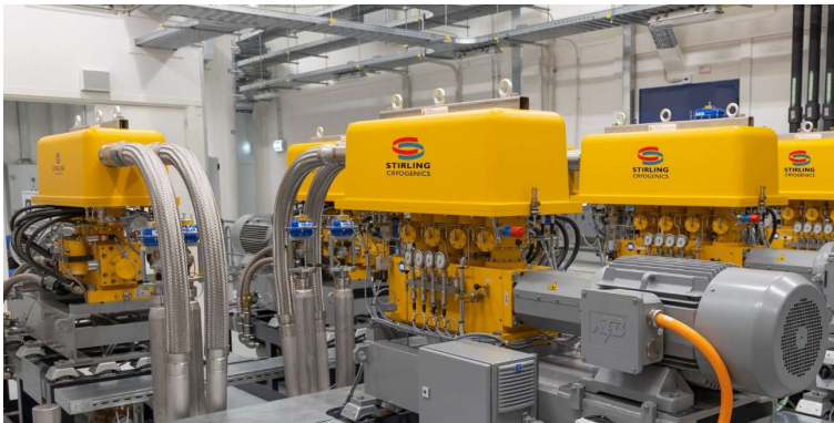
2019 Stirling Cryogenics Hydrogen Re-liquefier for Cold Neutron Source at RID Photo Courtesy Reactor Institute Delft, The Netherlands
